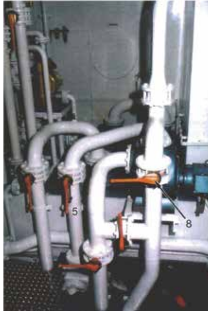
Fig. 7 - Ballast pump in the engine room, lines and (stop) valves
